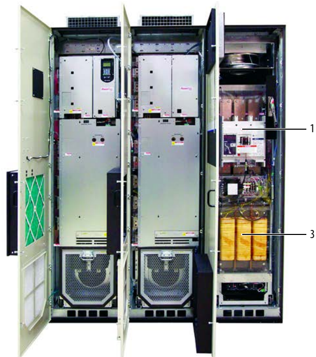
Input power landed behind circuit breaker, which is accessed by extracting rollout chassis.
