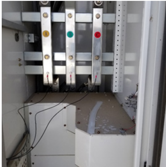
Inverter terminations show the PESD leads connected at the Load side of the 480V AC Bus.
