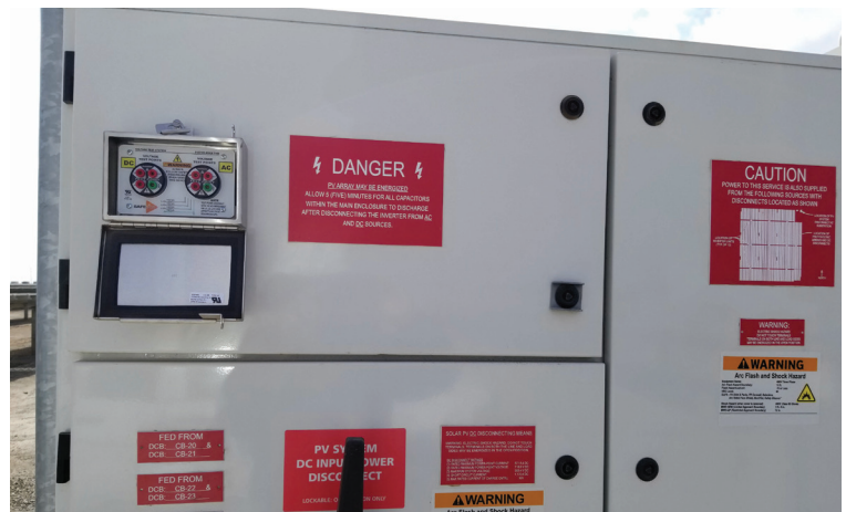
Two Safe-Test Points™ in Stainless Steel housing used to verify the absence of voltage on Line and Load side (DC/AC) of an inverter system in a PV solar application.
