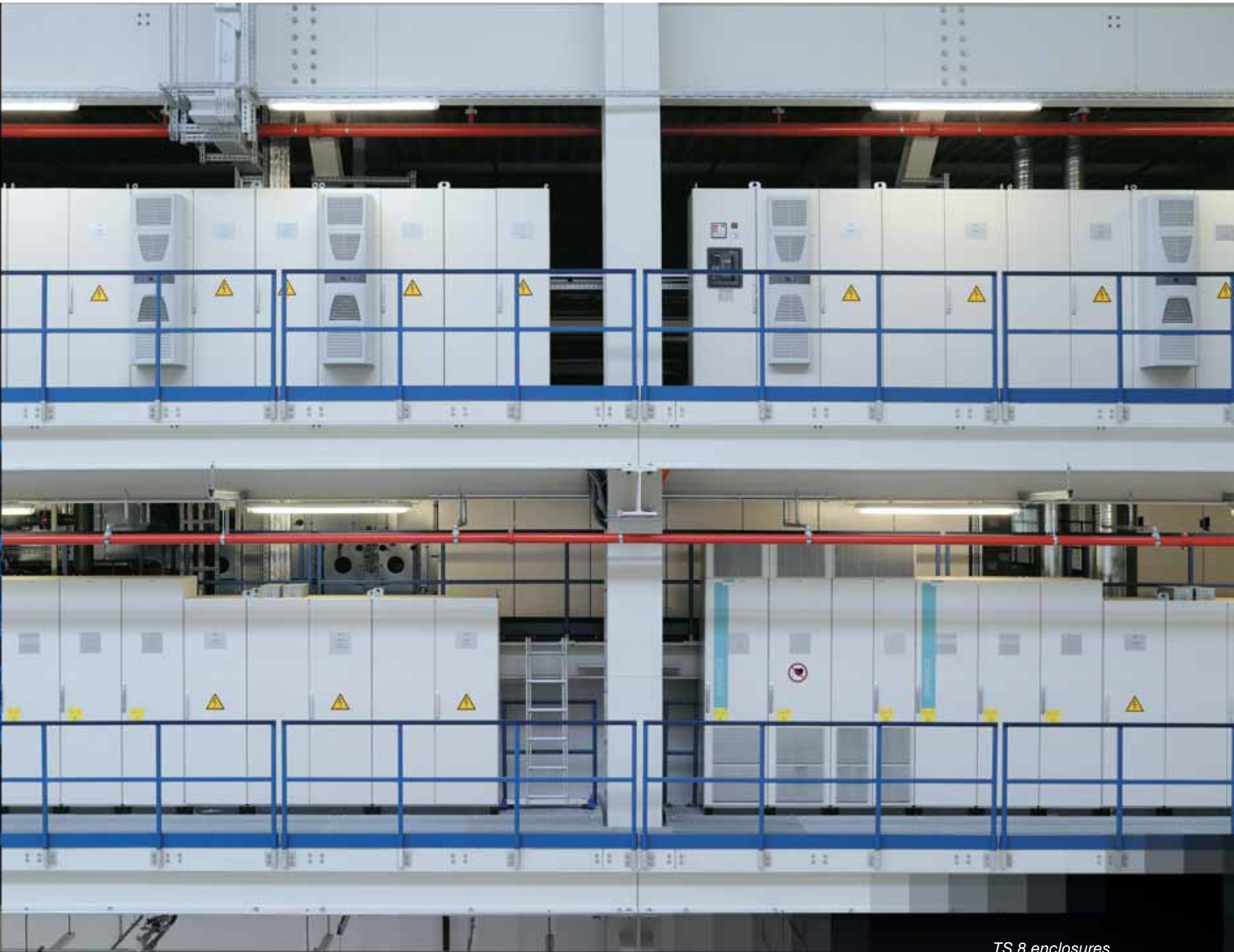
TS 8 enclosures in a car plant
