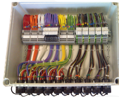
Terminal Distribution Box
